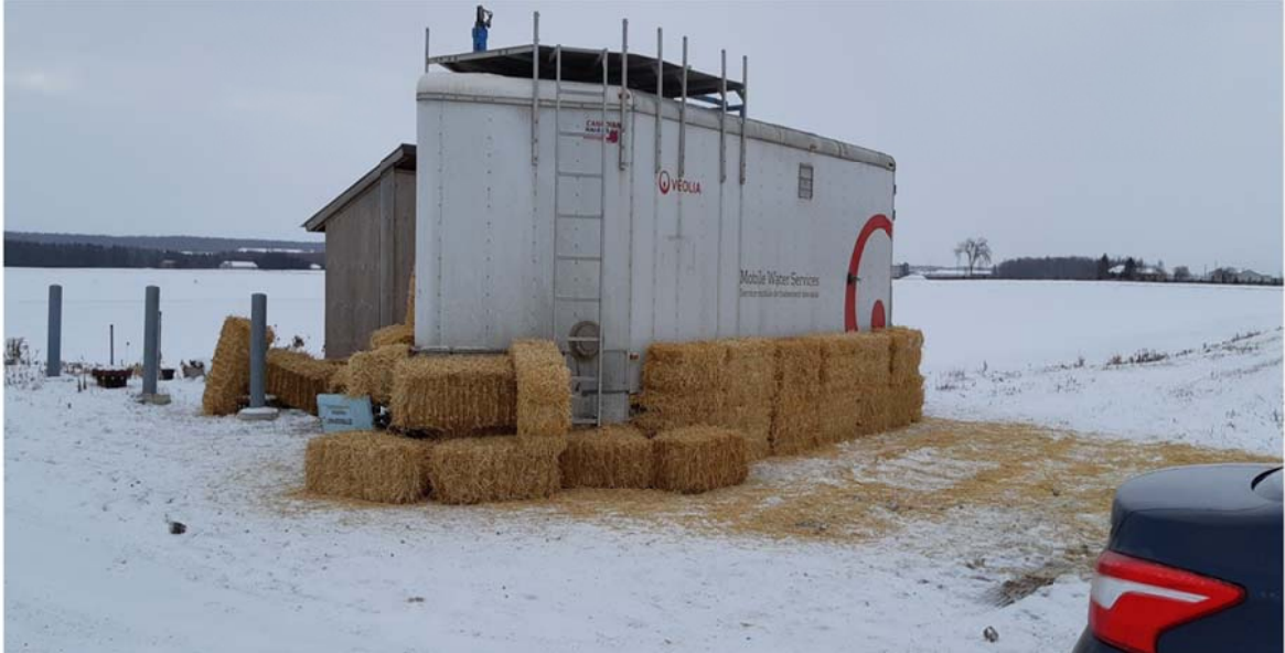
Figure 3-2 Exterior view of the LagoonGuard™ pilot unit with insulation
