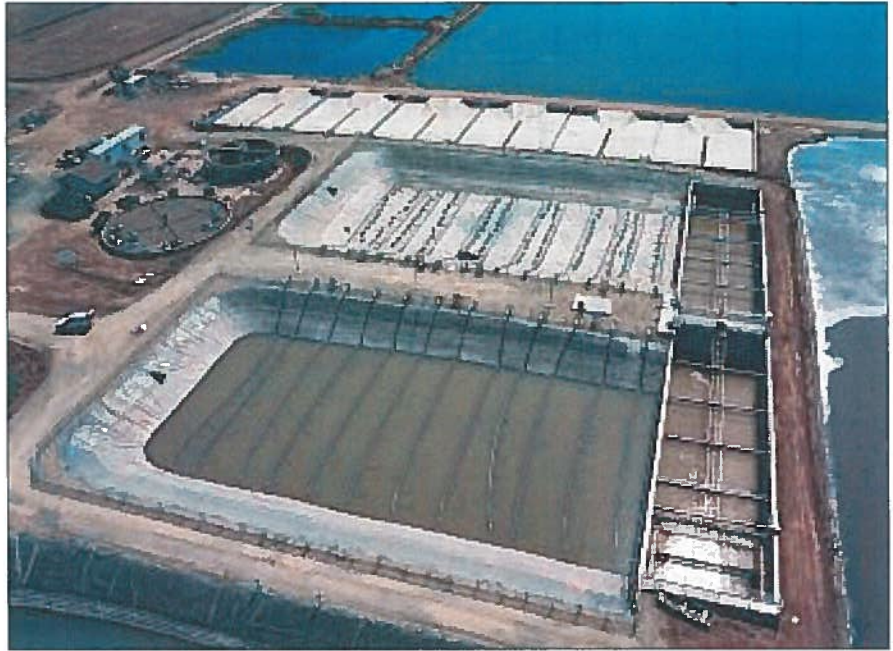
Biolac® basins with rectangular, flat bottom clarifiers under construction in California. Each clarifier will be fitted with Parkson's SuperScrapper® Sludge Removal System and SuperSkimmer Scum Removal System.
